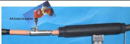
Figure 11: System of connecting cables at side
