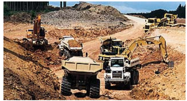
Figure 11. Picture of the new rail track Köln – Rhein-Main (Photo: Arge Mittelstand NBS)
