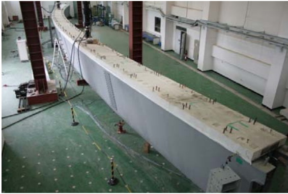
Figure 18. Overview of integration of trapezoidal open steel box girder and precast decks
