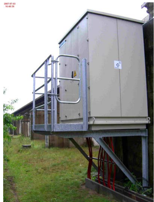
Figure 3: Compact switch station mounted at a guideway column
