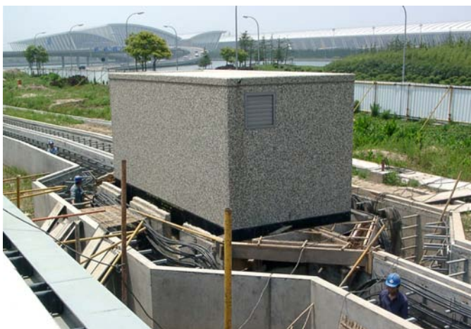
Figure 2: Switch station and cable tray on the Shanghai track
