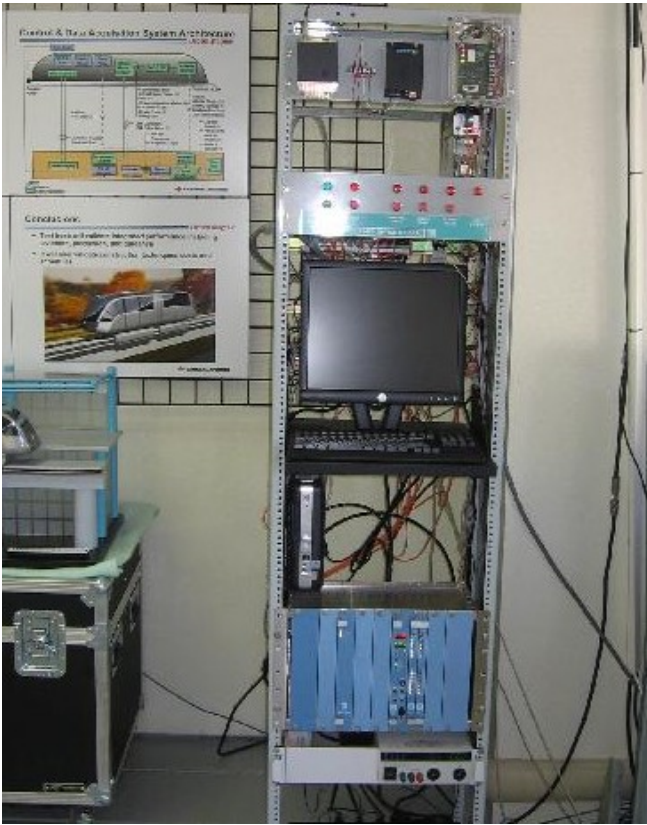
Figure 7: Control room equipment rack
