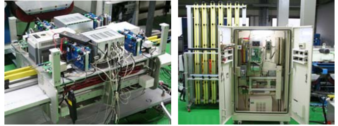
Figure 12 Pictures of STMAG and Non-Contact Power supply.
