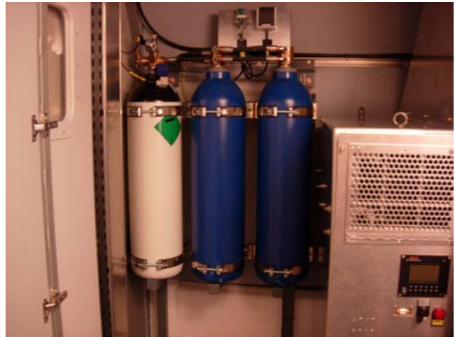
Figure 10. TR09 fire fighting system, pressure bottles
