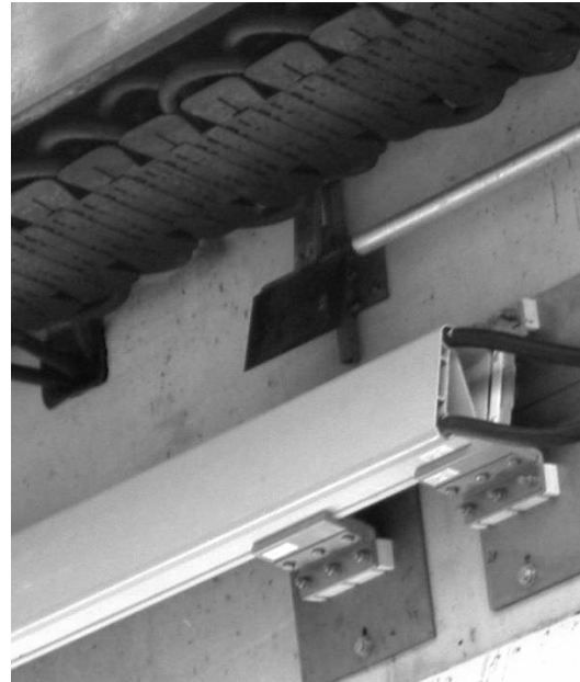
Figure 4: Primary cable support made of GRP on the Transrapid Test Facility Emsland.
