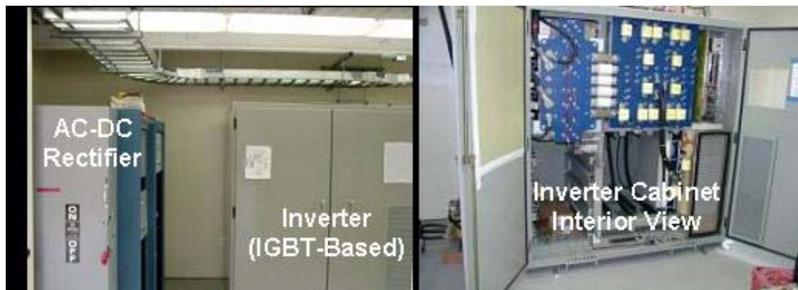
Figure 8. View of electrical room, which houses the rectifiers, variable frequency inverter, and train protection equipment
