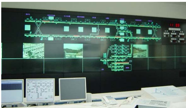
Photo-6 Train Operation Control Center (Refer to Photo-5.)
