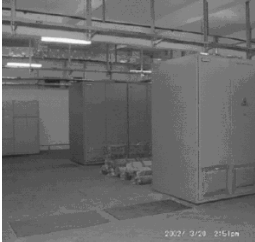
Figure 9: View in the converter room in Pudong Airport substation
